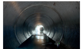
Sewage ducts and shafts
